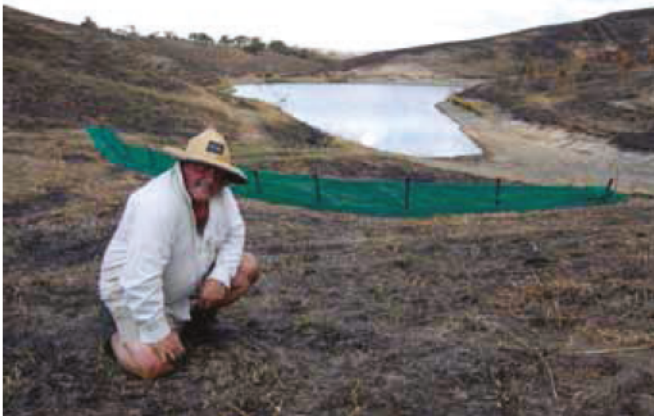
Figure 5.1: Sediment fence built to protect dam from debris and pollution after fire.
